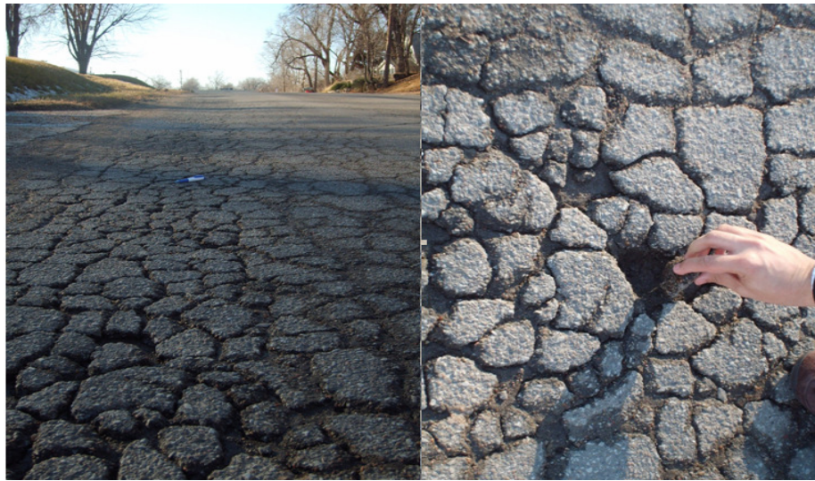
Figure 2.17 - Fatigue damaged pavement in Lincoln, NE
