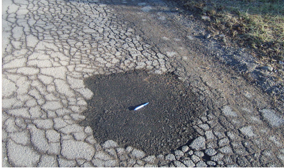
Figure 2.18 - Pothole created as a result of severe fatigue in Lincoln, NE
