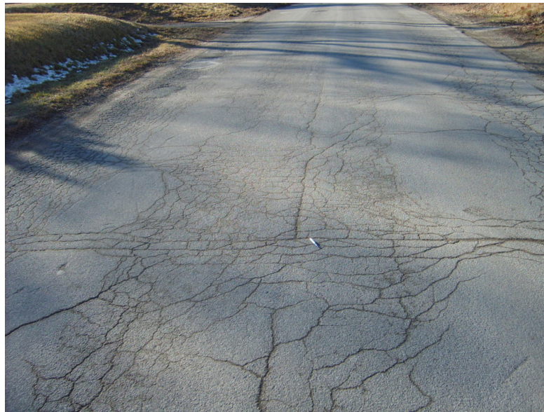
Figure 2.16 - Distresses of a low traffic pavement in Lincoln, NE
